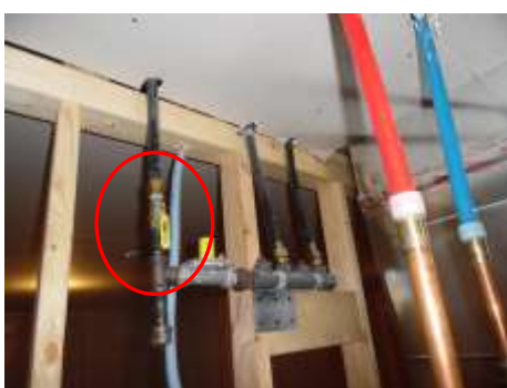
Gas plumbing shutoff location
