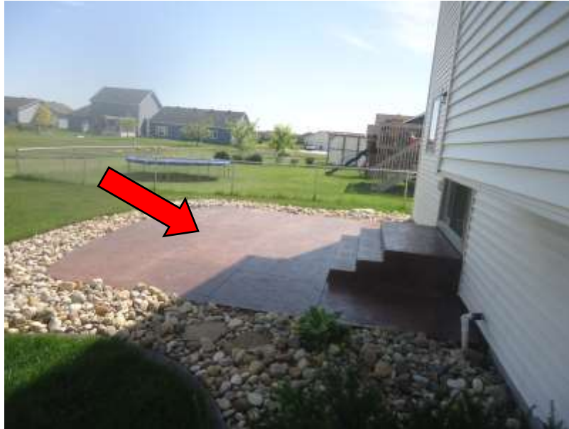
Patio was pitched toward the home. Maintain positive drainage away from the home.
