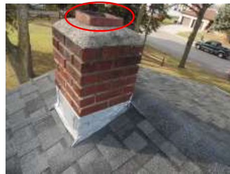
Recommend capping chimney with screened weather cap
