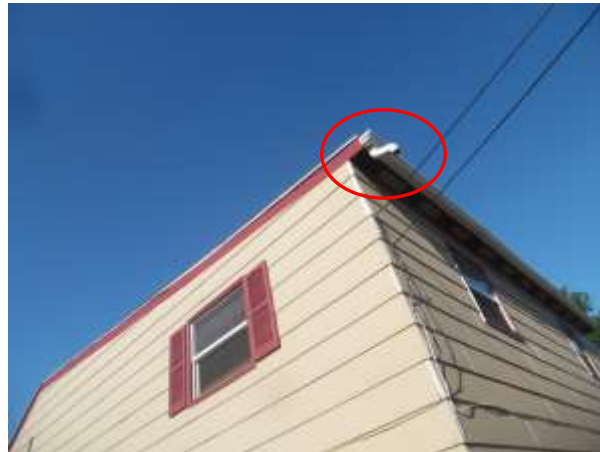
Downspout extension missing on gutters.
