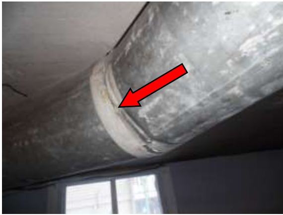
Asbestos like wrap on ductwork
