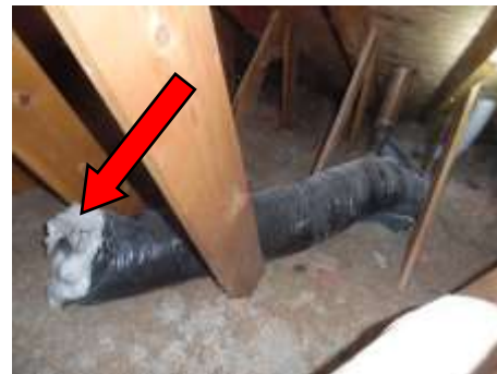
Bathroom exhaust fan discharged into attic.
