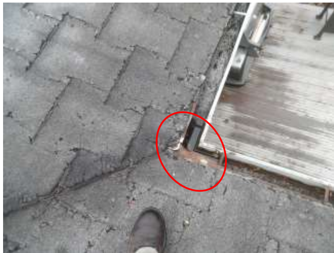
Visible portions of valleys/flashings had rusting/damage. Recommend replacing.
