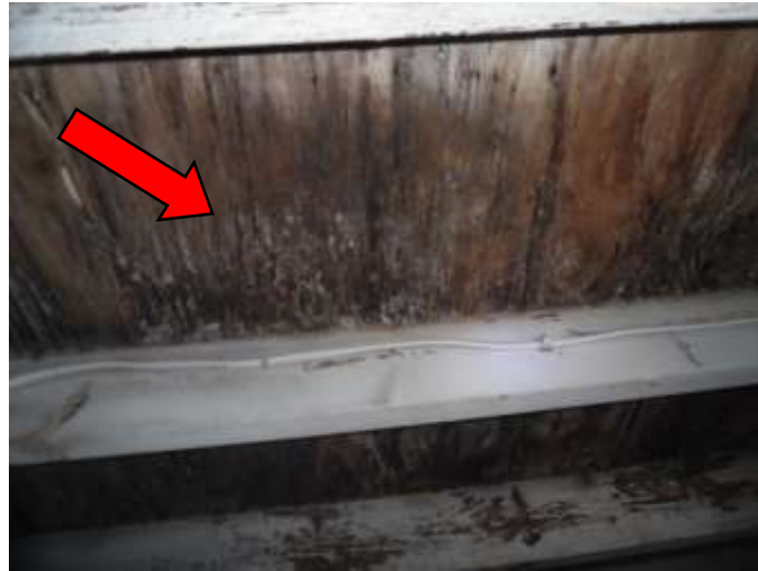
Mold like substance present on roof sheathing visible in attic.
