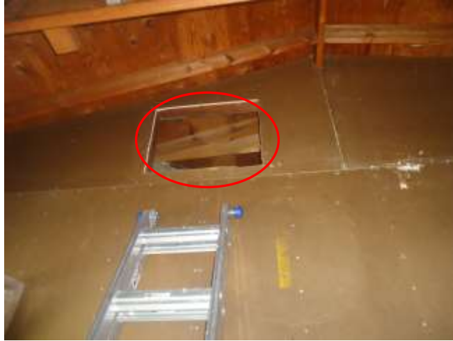
Attic hatch is a part of the firewall. Safety hazard!
