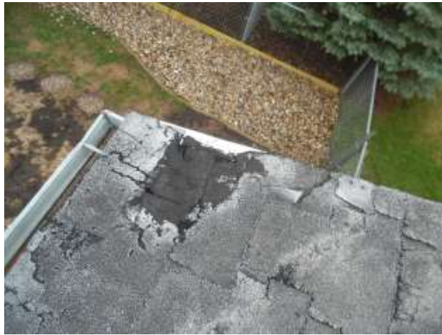
Roof had damaged area. Missing/damaged shingles.
