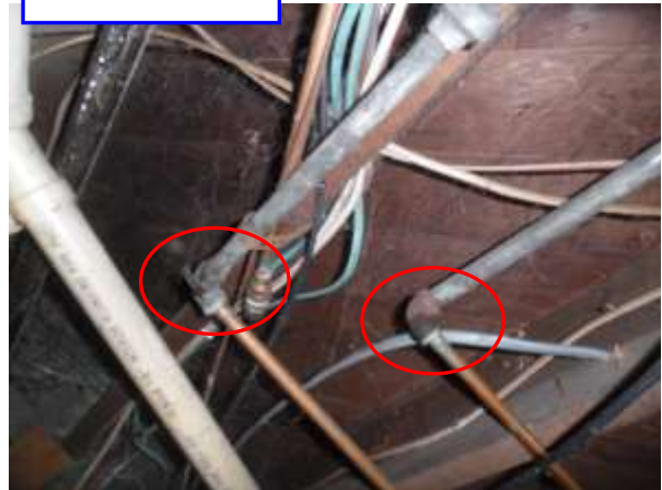
Plumbing had dis-similar metals connected.
