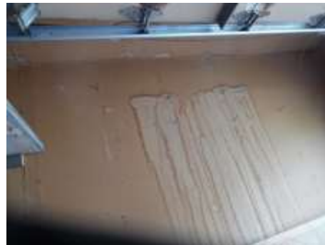
Moisture damage on garage drywall.
