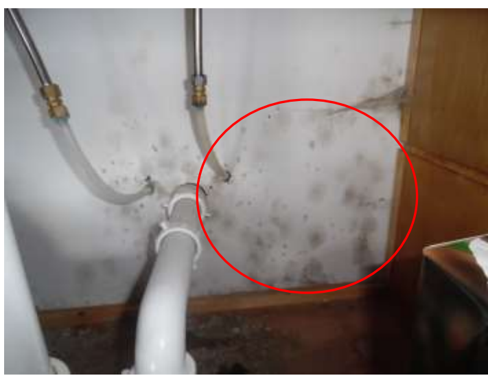
Mold/mildew like substance present under kitchen sink
