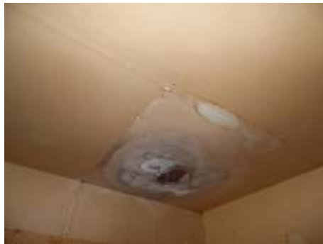
Moisture damage on garage drywall.
