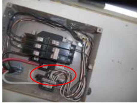
Sub-electrical panel in garage did not have proper neutral/ground separation.
