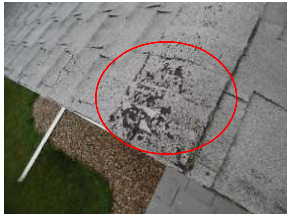
Roof had wear and damage with missing granules.
