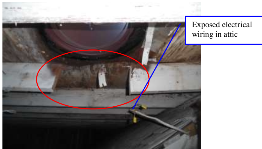
Cut rafter in attic.
