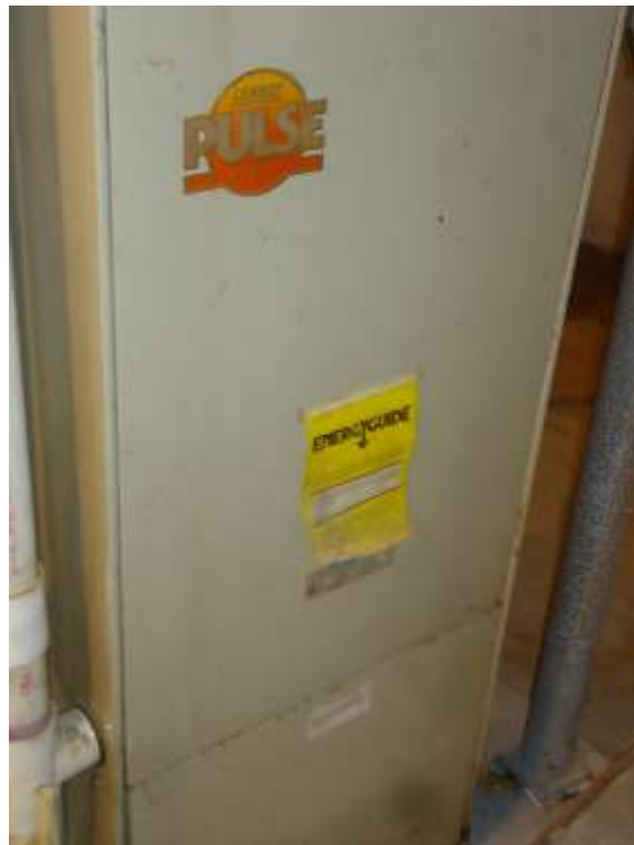
Lennox Pulse furnace - Have pressure tested
