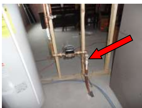
Water plumbing shutoff location
