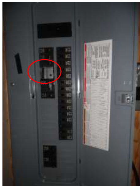
Open breaker slots in main panel. Safety Hazard!
