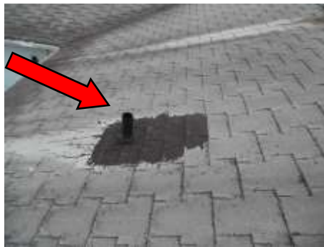
Flashings on plumbing vents had been tarred over.
