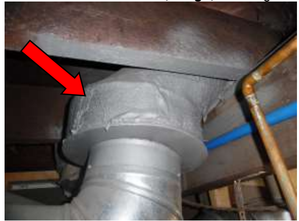
Asbestos like wrap, covered in mastic
